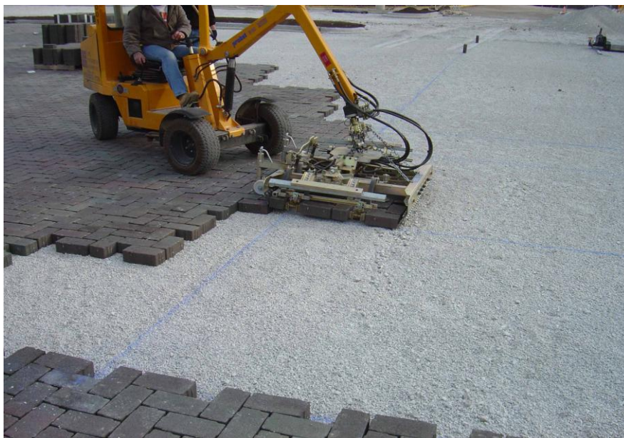
Figure 6. PICP units can be installed any time of year using mechanized methods. Photo courtesy of ICPI.
