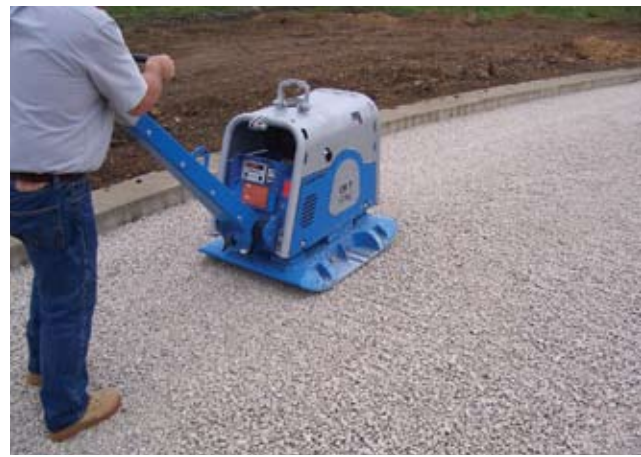
Figure 5. A 13,500 lbf (60 kN) plate compactor includes a device that indicates when no further compaction is needed on the area being compacted. This can reduce compaction time and increase assurance that the PICP open-graded base is compacted.
