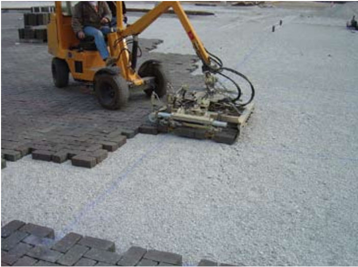
Figure 4. Many PICP projects are mechanically installed thereby decreasing construction time and labor costs because many pavers are placed at the same time.
