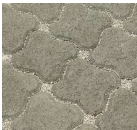
Figure 3. Left to right: After excavation, PICP construction begins with placing and compacting an open-graded subbase and base as shown in the first two photos. The next photo shows mechanical installation of the concrete pavers on a screeded bedding layer of small aggregate. The rightmost photo illustrates small aggregate in the openings and joints that enable high surface infiltration. The pavers and aggregate are compacted to create an interlocking pavement.
