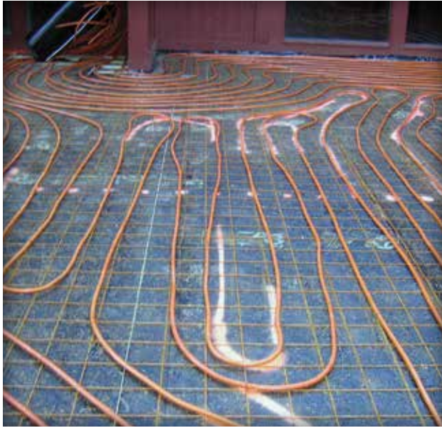
Figure 4. Pipes for a hydronic (liquid) heating system are placed on wire mesh and fastened to it with plastic ties prior to spreading the bedding sand and installing the pavers.
