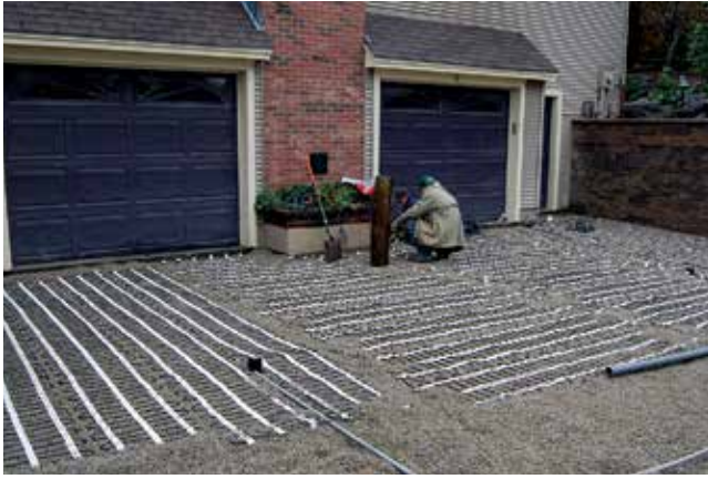
Figure 10. Electric heat tape snow melt system is installed in the bedding layer of permeable interlocking concrete pavement.
