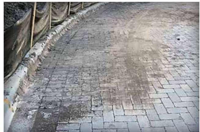
Figure 3. Whether eroded onto or dumped on PICP, erosion and sediment control are essential during construction.
