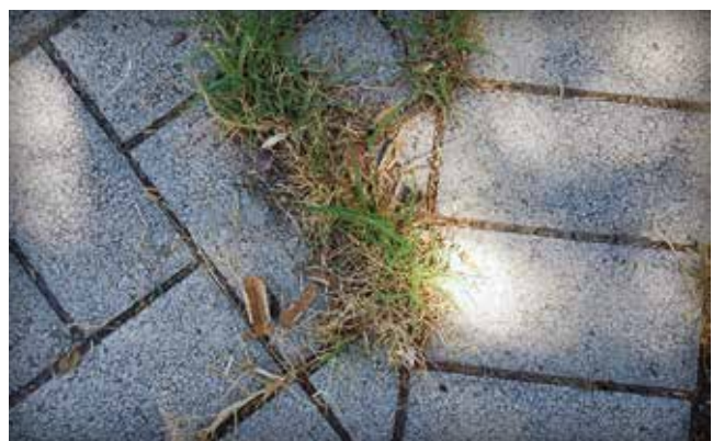
Figure 9. Weeds indicate sediment accumulation and lack of surface cleaning to remove it.
